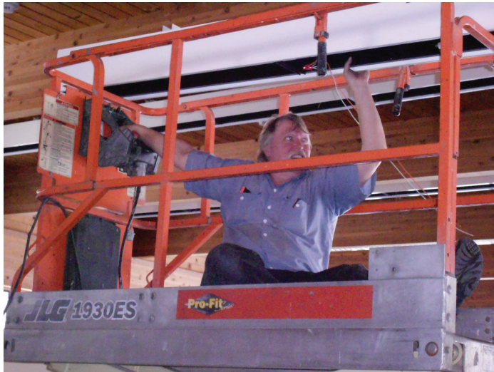
A lift was needed to complete removal of the old lighting fixtures, as demonstrated by Mike Lund
